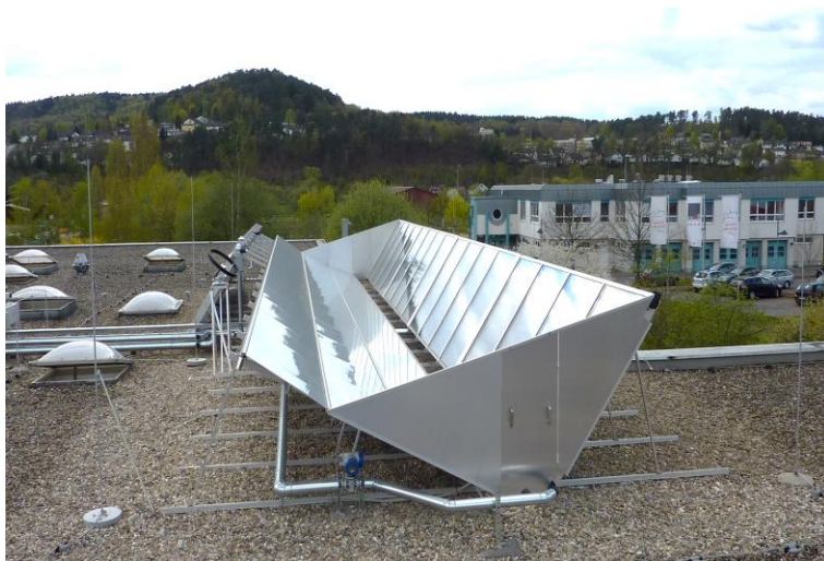
Figure 1.3: RefleC prototype at pilot plant laundry Laguna in Marburg an der Lahn
