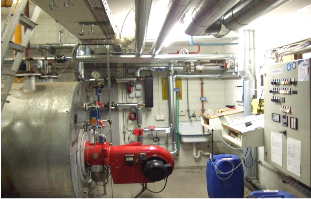
Figure 5.3: Boiler room with one of the initially two steam boilers on the left hand side, its gas burner (red, foreground), and the boiler control board (right). In the central back-ground, a plate heat exchanger for solar pre-heating of the boiler feed-water is visible (black insulated). Below is the changeover valve for solar pre-heating of the discharge loop before the heat exchanger is flown through (red with red LED). A ladder (left) leads to an intermediate story above, where the boiler feed-water tank is located.
