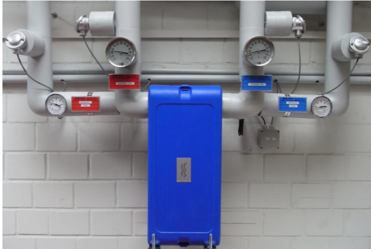
Figure 5.10: Plate heat exchanger for solar pre-heating of the boiler make-up water. Four Pt 100 temperature sensors measure the temperature differences at the primary side (discharge loop) and the secondary side (make-up water pipe) of the heat exchanger.
