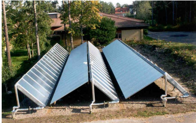
Figure 1.13: Flat-plate collector field with trapezoidal corrugated aluminum sheet booster reflectors supplying a hospital in Östhammar, Sweden.
