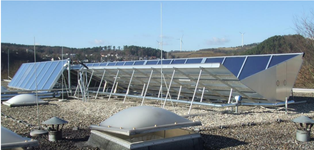
Figure 5.4: Collector field of the pilot plant from east direction. On the right, the eastern of the two vertical RefleC trough closure reflectors (with revision opening) is visible. Three pyranometers are located centrally in the field beside the front row. One of the MIDs (magnetic inductive flow meters) can be recognized in the right field inlet pipe (light blue cover). The vertical stakes belong to the lightning protection concept.
