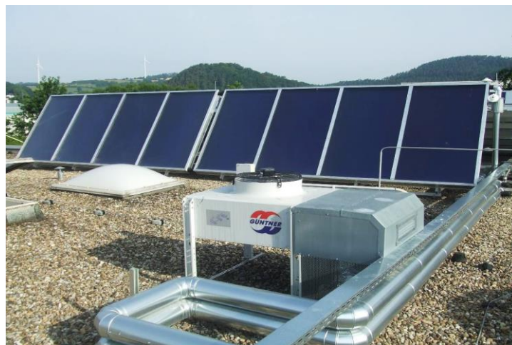
Figure 5.8: Dry stagnation cooler in front of flat-plate subfield. The insulated and aluminum sheet metal coated feed and return flow pipes of the field are routed in a U-shape to compensate thermal expansion. Above them, the rectangular sensor cable duct is visible.
