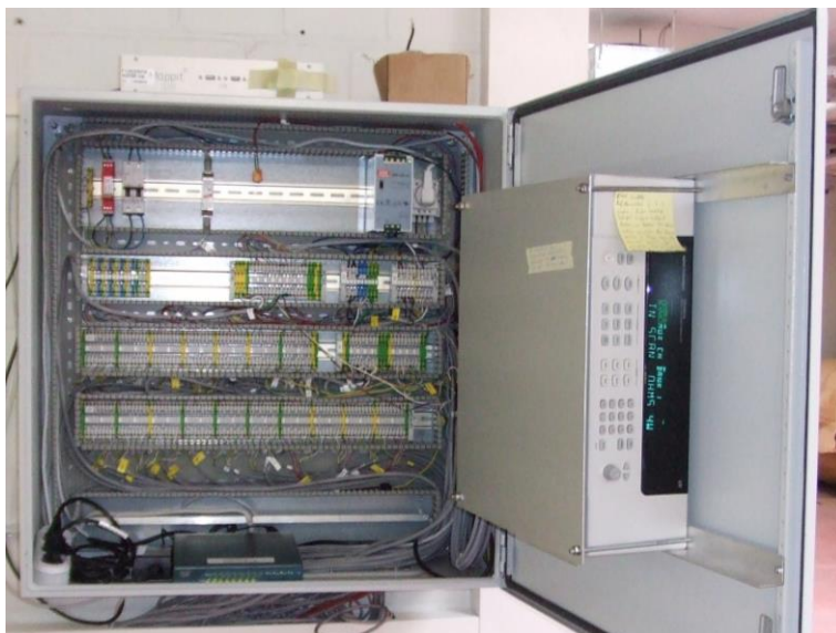
Figure 5.11: Monitoring switch cabinet with cable ducts opened. The large box at the cabinet door (right) is a multiplexor, logging sensor signals. The Linux-PC placed on top of the control cabinet processes the signals and transfers the daily data file to a monitoring server of Fraunhofer ISE via the hardware-firewall ASA (Advanced Security Appliance) placed inside at the bottom of the control cabinet.
